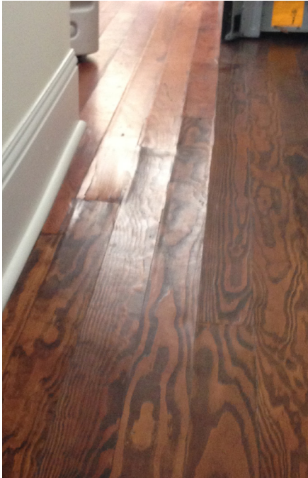
Wood floors can ‘cup’ while curing and should be dried out slowly after a flood.
