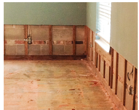
It is easier to relocate electric outlets to reduce future flood damage when wall finishes are removed and repaired.
