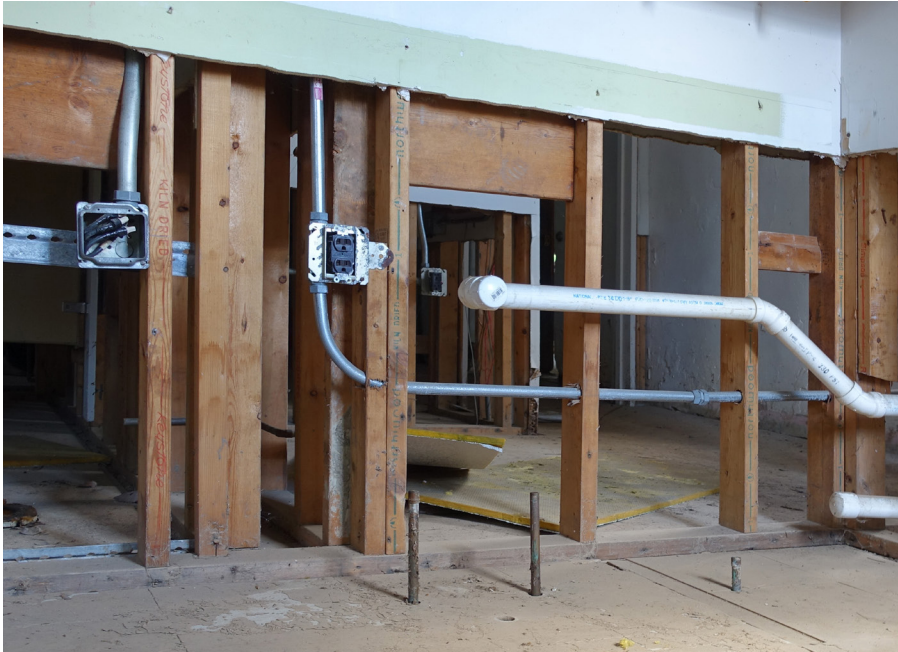
A significant remodeling project can provide an opportunity to elevate electrical and plumbing components to improve resilience.
