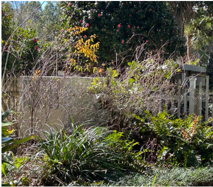
The generator is highly obscured by fencing and surrounding plants.
