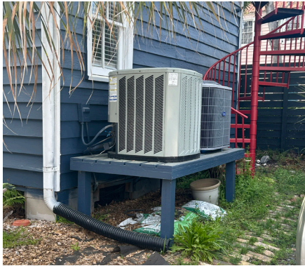
Stands for elevating equipment can be purchased or made from lumber at home. Stainless steel or galvanized connectors will limit rusting.
