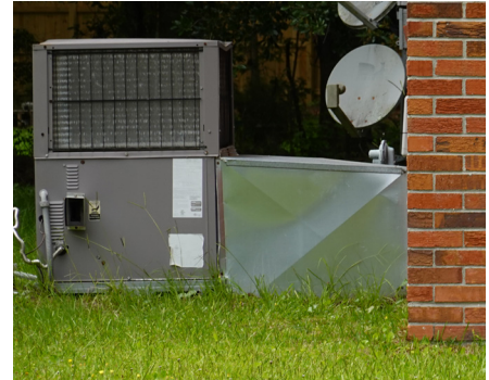
Package-style HVAC systems require more space and exterior ductwork at ground level, which can complicate system elevation. Ducts in flood-prone areas are vulnerable to damage.
