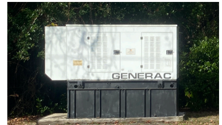
Generators can be installed as a permanent system that is ready to use when there is a power outage.
