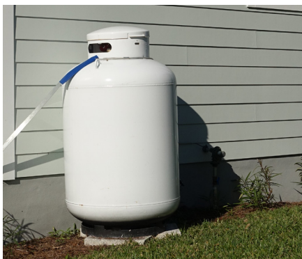
Secure propane tanks to reduce movement during a flood or earthquake.
