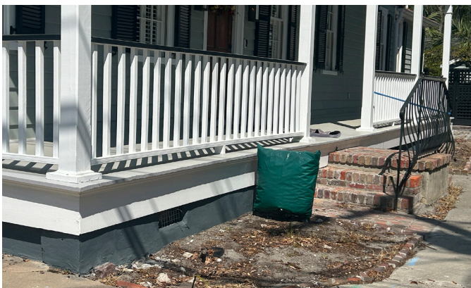
The backflow preventer, disguised by the green cover, keeps floodwater from backing up into drains and plumbing fixtures.
