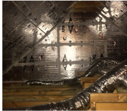
Relocate ducts to attic, above potential floodwater. Installing new insulated ductwork will increase system efficiency. ( www.energy.gov )
