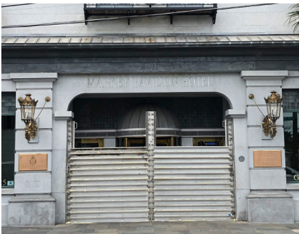
Flood panels installed for preparation of an upcoming flood event. (Courtesy of Glenn Keyes)
