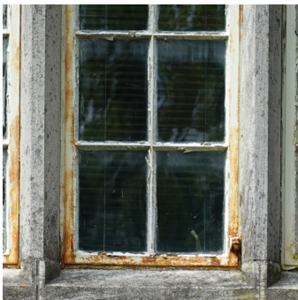
Steel windows can rust, requiring cleaning and rust-inhibitive primer and paint.
