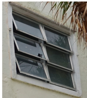
Aluminum window sashes can be easily bent allowing air and water to enter.
