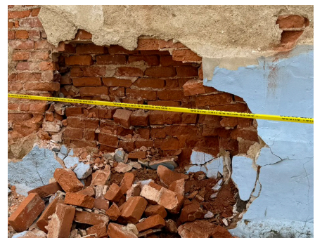
Consult with an architect or engineer for severe cracks or partial collapse of masonry walls.
