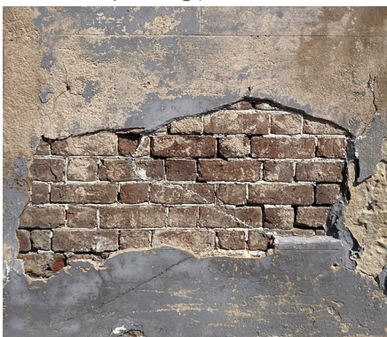
The loss of a stucco coating from a masonry wall can allow water to be absorbed by the underlying masonry, advancing deterioration of the brick and mortar joints.
