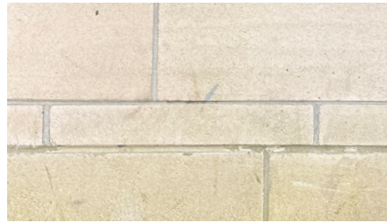
There is a wide range of stone types, colors, and coursing patterns. Regular maintenance of mortar joints is critical.
