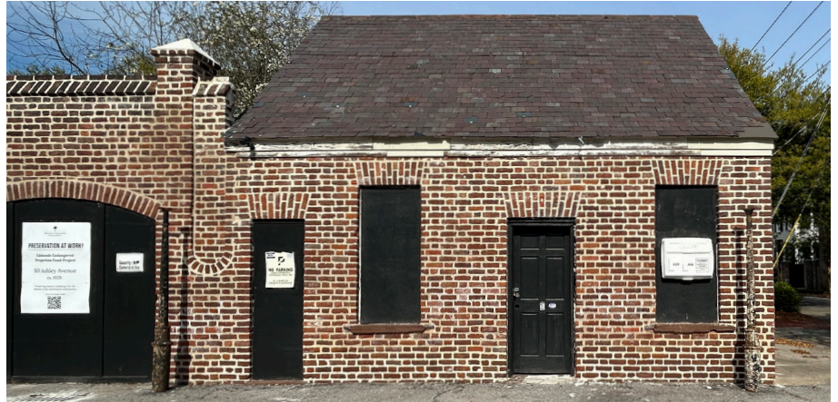
Buildings should be stabilized and secured while awaiting rehabilitation.
