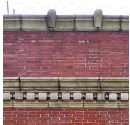
Terra cotta can flake or spall allowing water and wind to penetrate into structural components.
