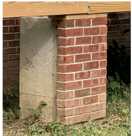
A full-width brick veneer has been installed on this new poured concrete pier at a building elevation to mimic the original appearance.
