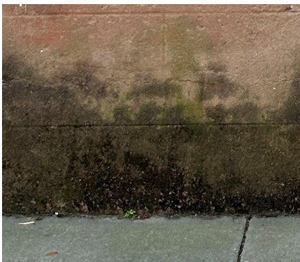
The algae along the foundation suggests significant moisture in the wall. Possible sources can be pooling adjacent to the wall, rising damp, or rainwater splashing from the sidewalk.
