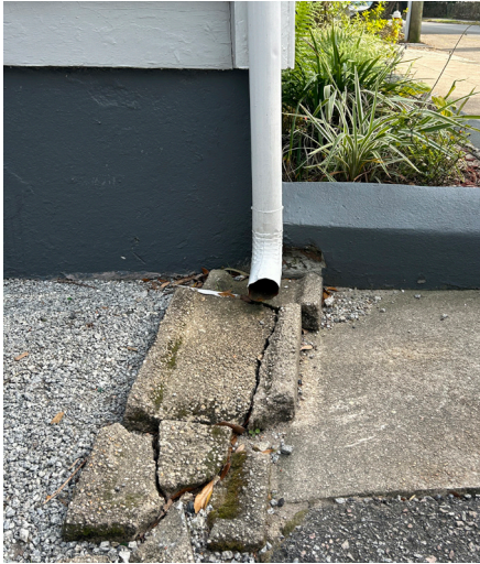
Avoid locating downspout discharges near masonry walls and foundations.
