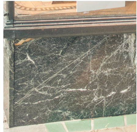
Marble or granite veneers are often applied at the apron under storefront windows on commercial buildings.
