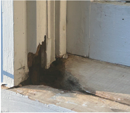
Deteriorated and rotted wood can be carved out.
