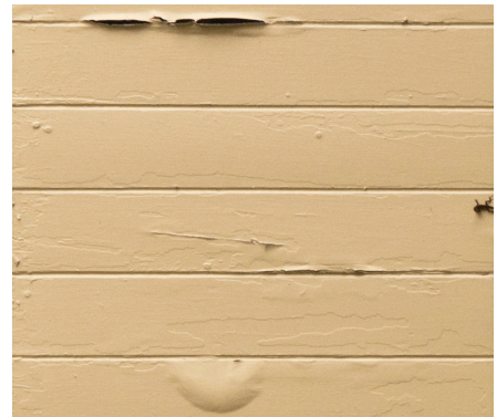
Paint can deteriorate over time or be an indicator of underlying problems that show as wrinkling, peeling, blistering, cracking or crazing, or alligatoring.
