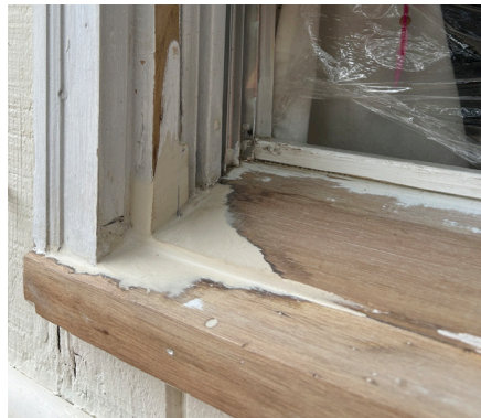
Epoxy has been applied to match the profile of the existing trim.
