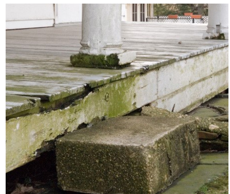
Wood that is in contact with the ground, situated close to plants, or in areas prone to splashing water are particularly vulnerable to rot and must be regularly cleaned and painted.
