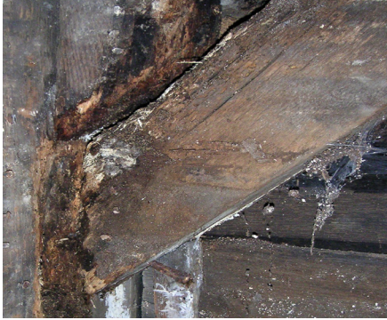
Exposed roof framing in the attic can have pest and moisture problems.
