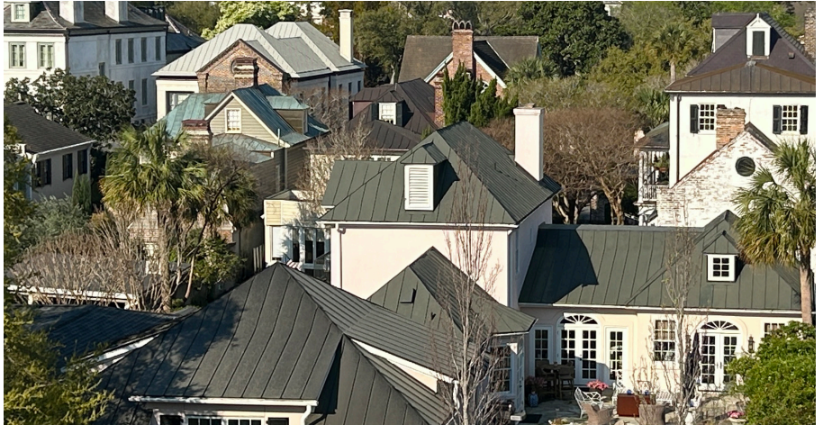
A roof may have one pitch or multiple pitches. All roof valleys, ridges, chimney or window joints, and eaves require proper flashing to prevent stormwater leaks.
