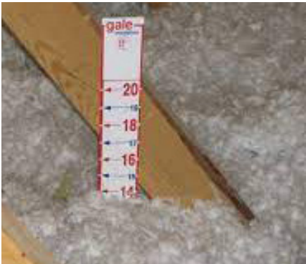
Loose insulation should be measured to monitor depth. (energy.gov)
