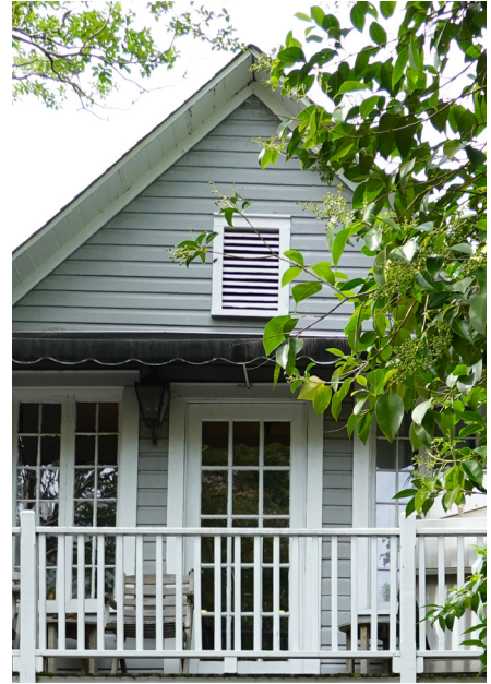
Any openings, including attic vents, will need temporary storm protection.
