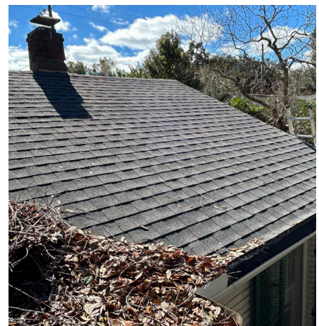
Leaves need to be cleared from the roof and gutters. A professional service may be needed to access the roof safely.
