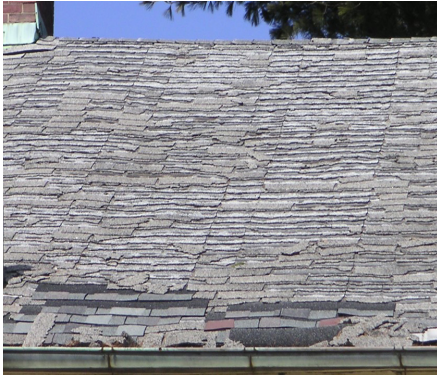
Individual shingles are missing and others are in a deteriorated condition.
