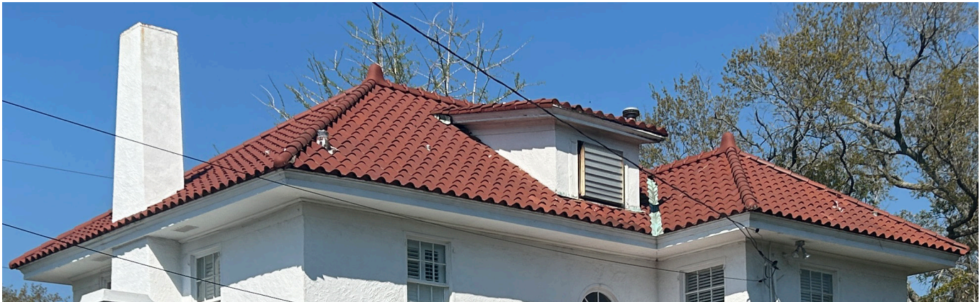
The roof eave projects beyond the building wall below. Eaves can be open, with exposed rafter tails, or boxed with vented spaces (as in this example).
