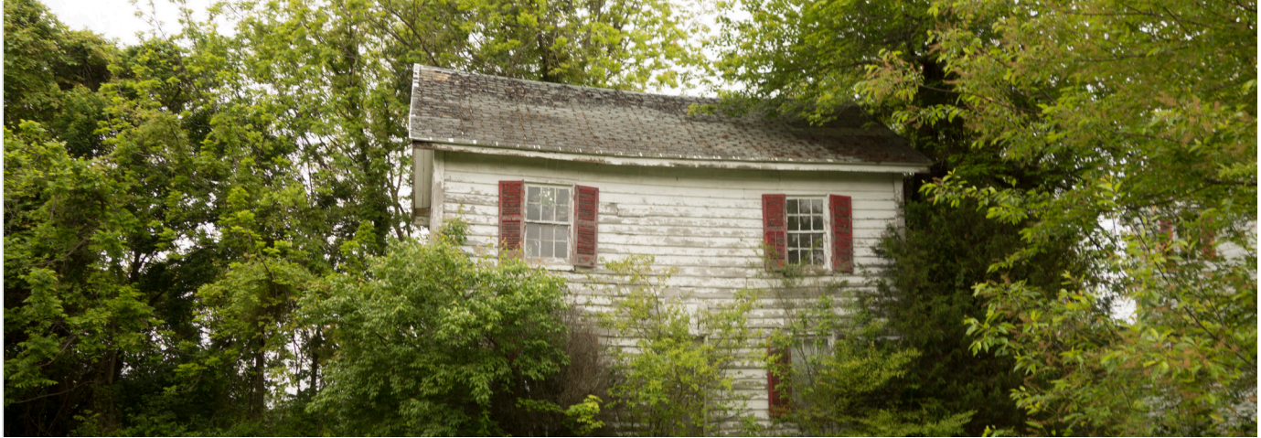
This roof needs shingle replacement and evaluation for structural repair. Overhead trees limbs should be trimmed so they are not touching the roof.
