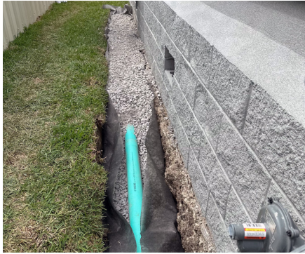
A French drain collects and moves water away from the foundation to reduce building water damage. (LSU Ag Center)
