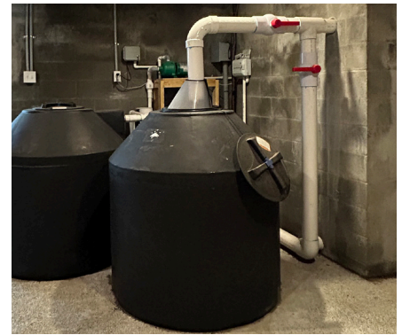
Cisterns provide larger storage capacity.
