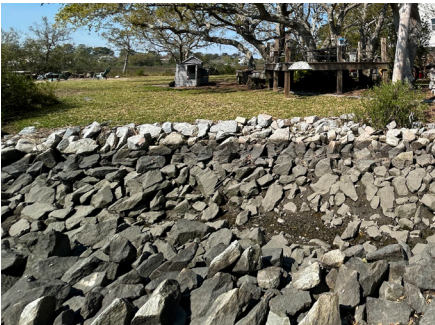
Stone and rock rip-rap can help stabilize the shoreline.
