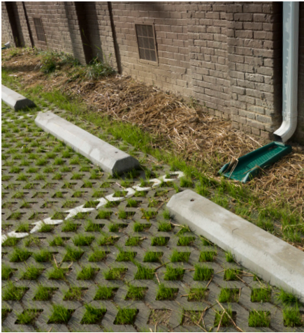
Open concrete pavers allow grass to grow in this parking area, which helps absorb more stormwater.
