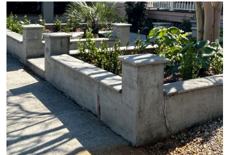
Low retaining walls can be used to manage a change in slope, control water flow, and collect stormwater to allow it to percolate.
