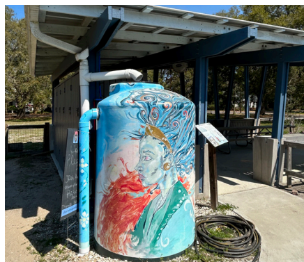
The roof downspout discharges into a rain barrel.
