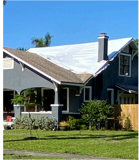
Wind damage to roofs can cause significant interior damage if water leaks occur.
