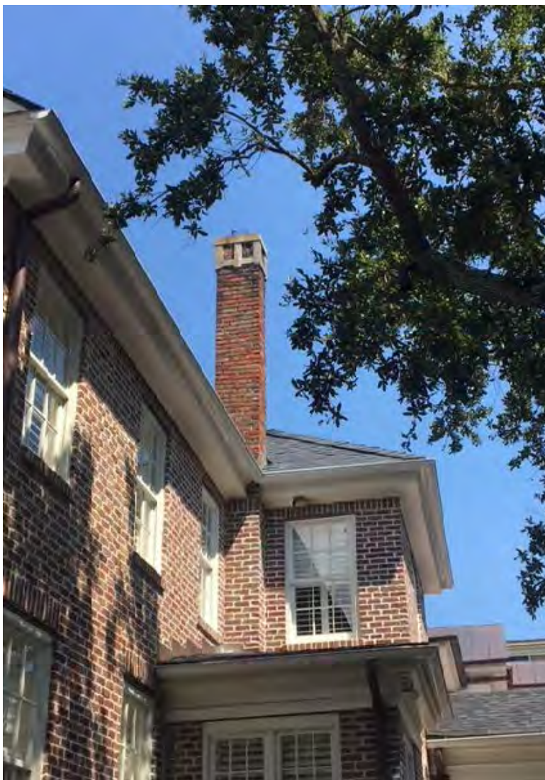
View of chimney at roof valley located at the intersection of the South and West elevations. Photo taken standing at backyard fence.
