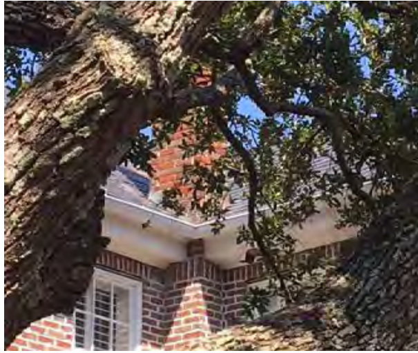
Detailed view of chimney situated at roof valley. Streetscape view of chimney is obstructed by tree.
