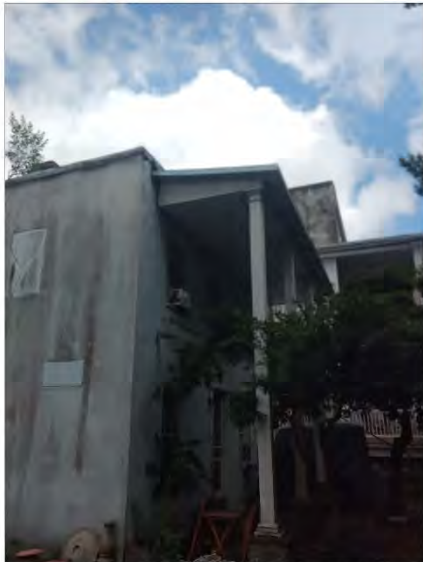
EXISTING GUEST HOUSE PORCH PULLING AWAY FROM STRUCTURE
