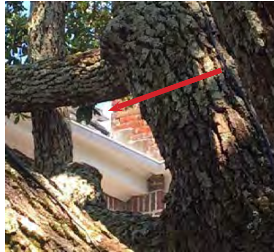
Detailed view of chimney situated at roof valley. Arrow depicts valley adjoining Northeast corner of chimney.
