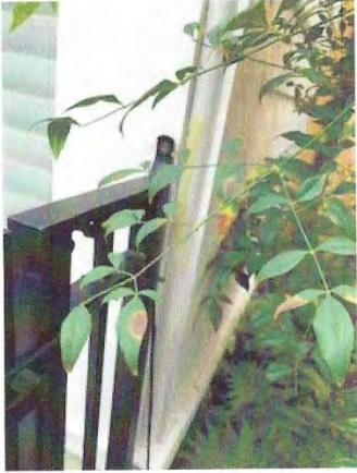
Window frame of Apt A cracking From stress from Apt B gate being Attached to Apt A
