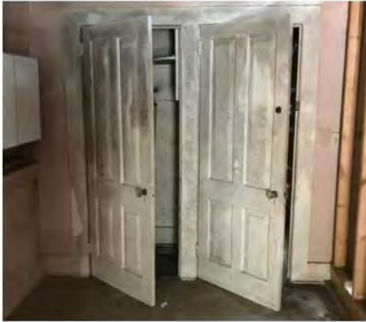
MOLD AT REAR ADDITION
