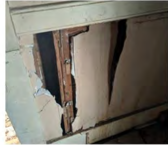
DAMAGE AT REAR ADDITION
