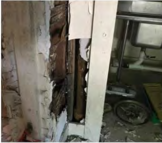
WATER INTRUSION DAMAGE AT REAR ADDITION
