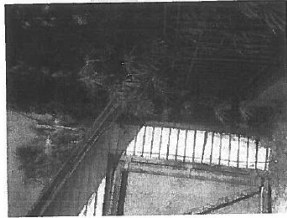
11. Right Side Exterior Stud Wall with Trees Adjacent to it (Not Accessible).
