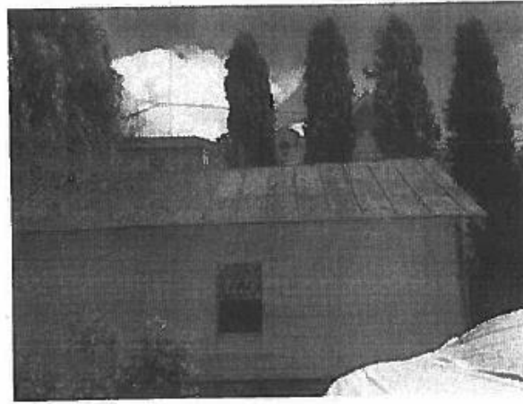
9. Metal Roof with Rust .
