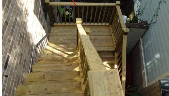
① CURRENT VIEW: NEW WOOD STAIRS- LOOKING EAST FROM TOP OF STAIRS
