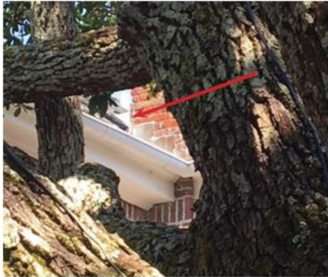
Detailed view of chimney situated at roof valley. Arrow depicts valley adjoining Northeast corner of chimney.
