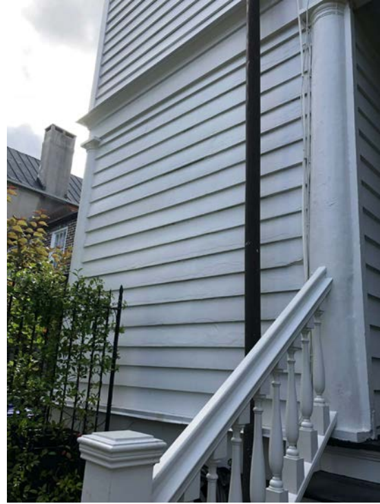
View from side yard looking north towards (south) side facade and area of proposed door and staircase.
