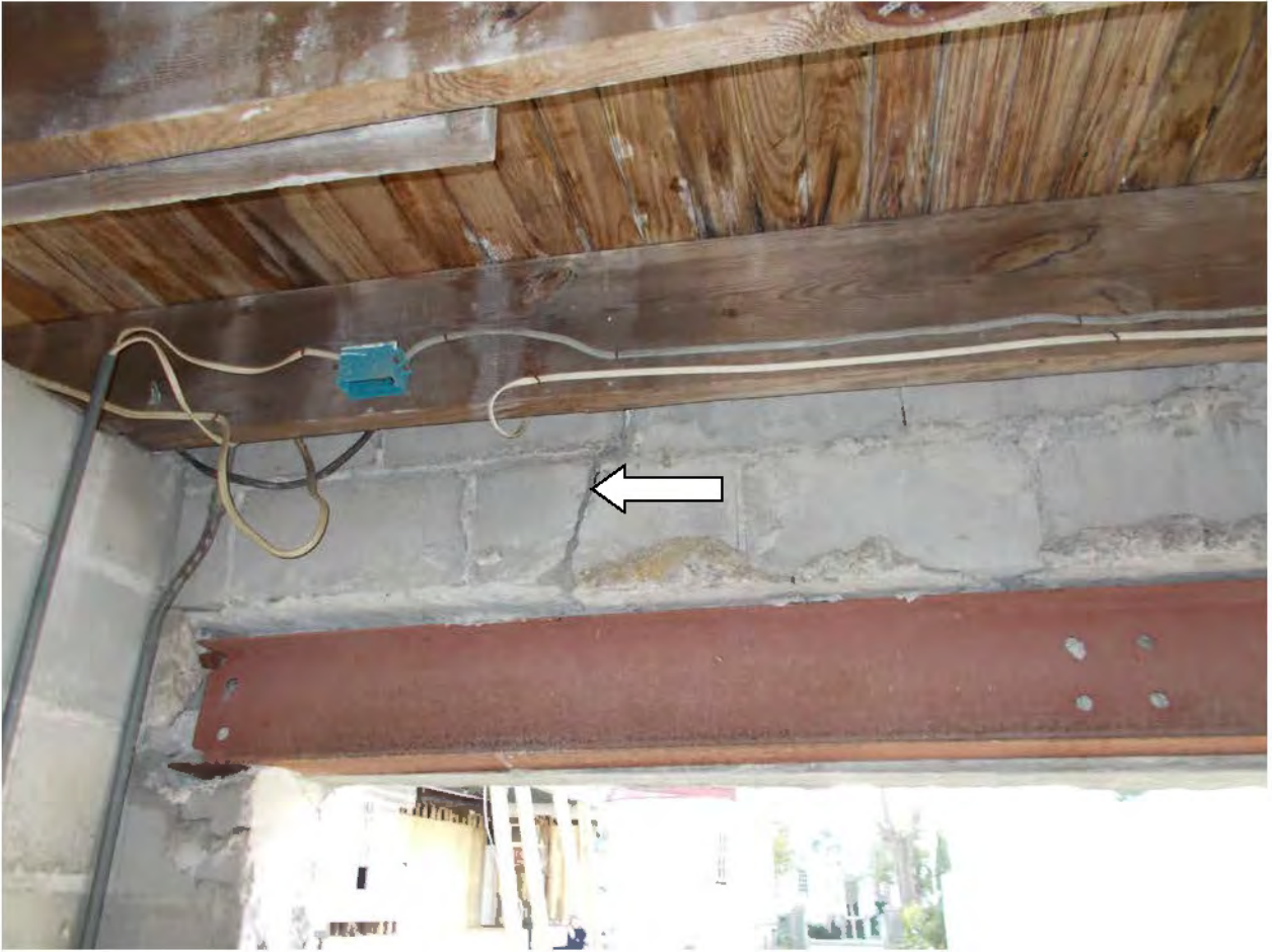
Figure 6: south side interior at the steel lintel. Note the 1/2" wide crack.
