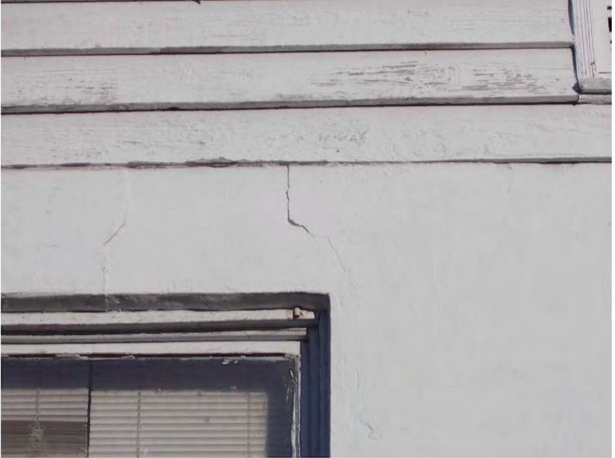
Figure 4: South side exterior cracks on the facade
