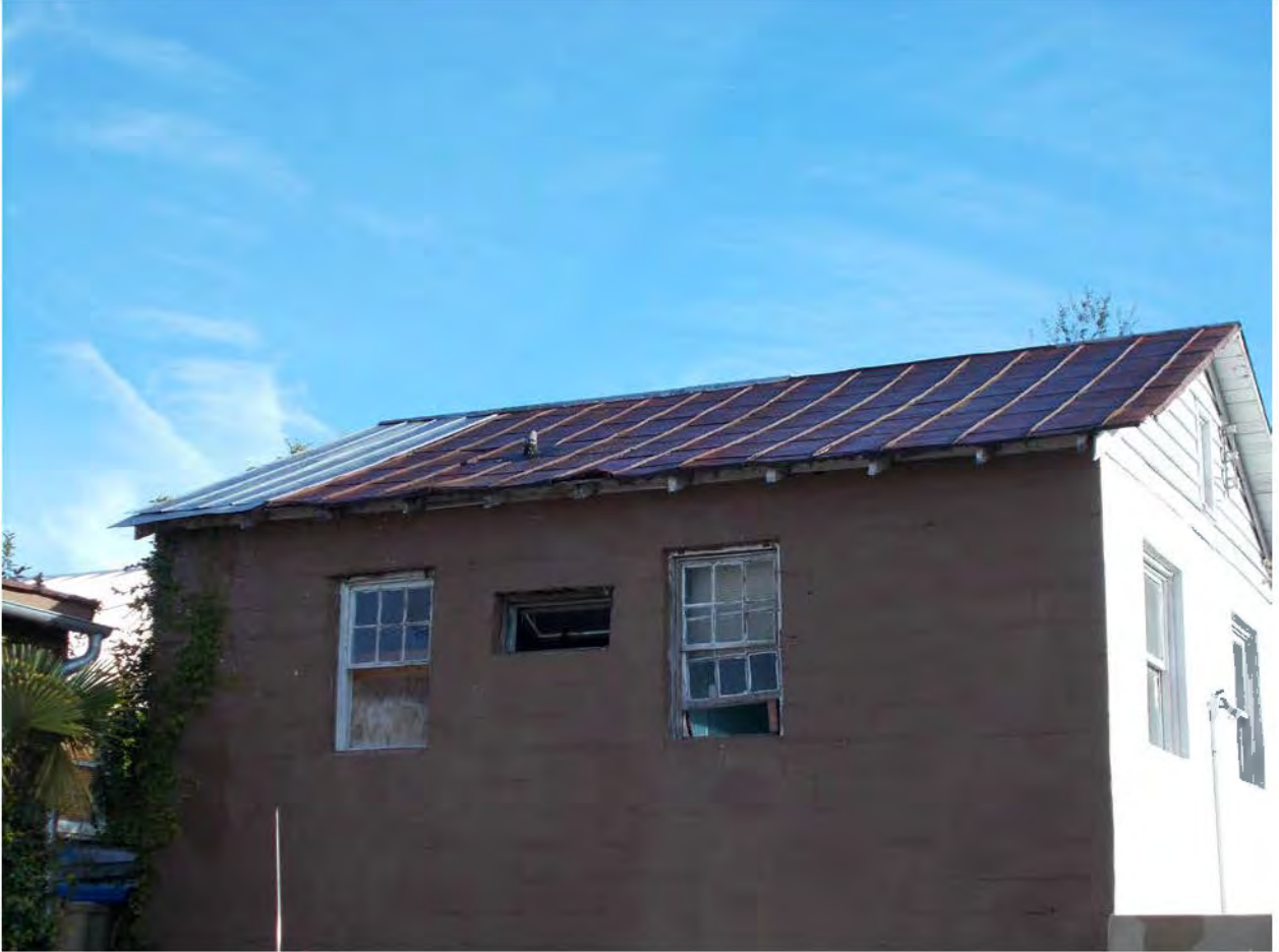
Figure 14: west façade, view of the roof. Note the metal covering rust, and the bow of the roof
