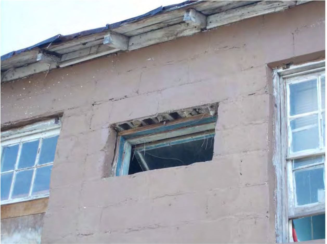
Figure 13: west façade, second floor. Note deterioration of the rafter tails and window surround.
