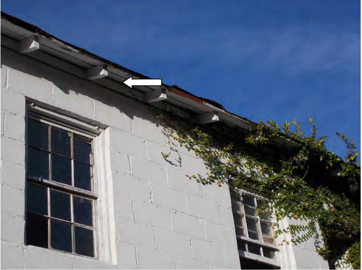
Figure 5. East side second floor exterior. Note the deteriorated rafter tails and roof sheathing.
