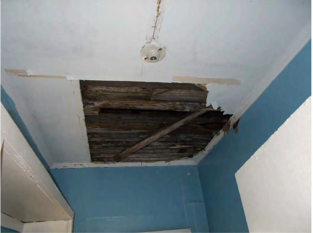
Figure 11: another example of west side second floor ceiling framing damage due to water intrusion
