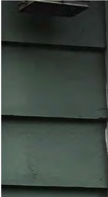
1 EXISTING LIGHT FIXTURE
