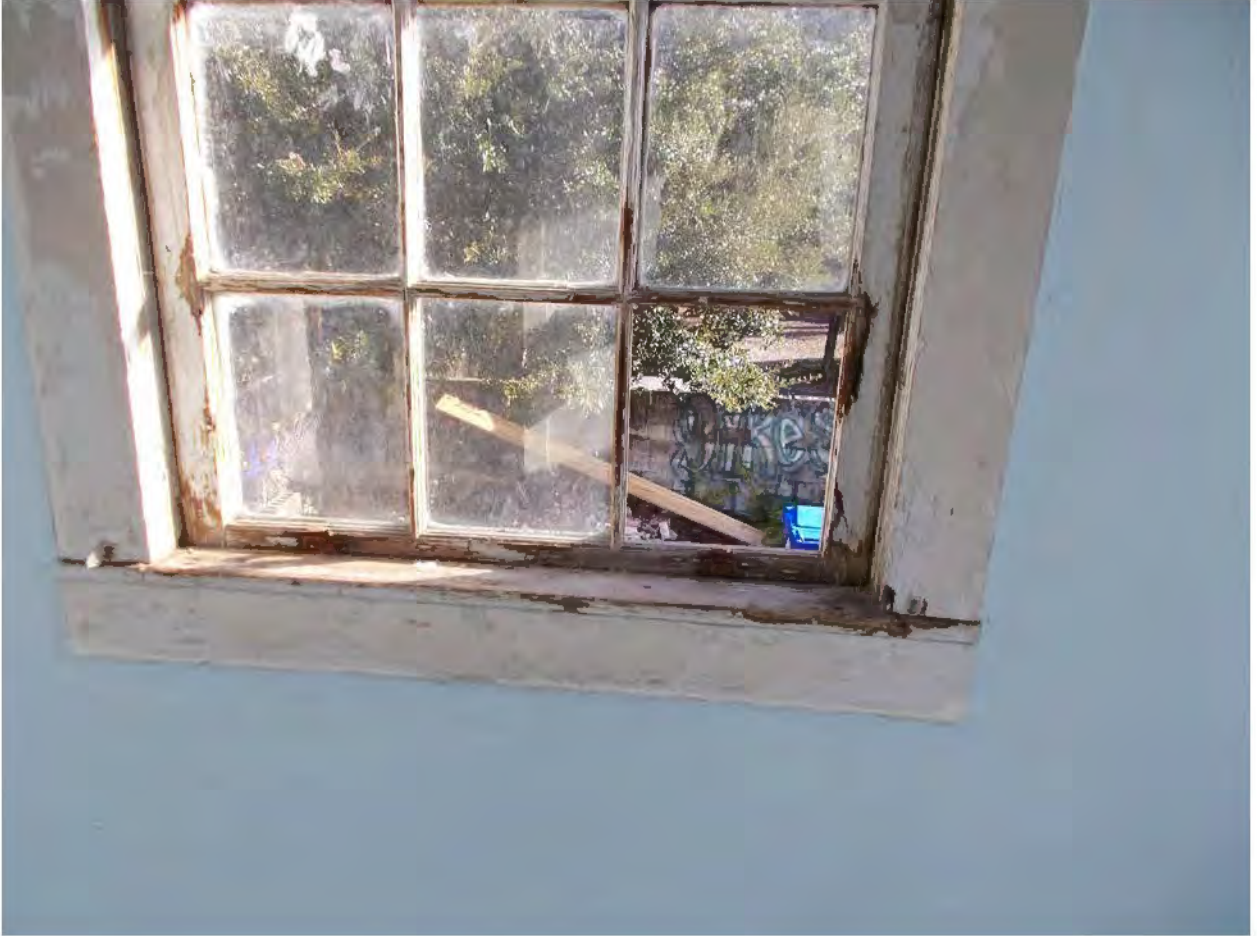
Figure 9: typical window surround deterioration
