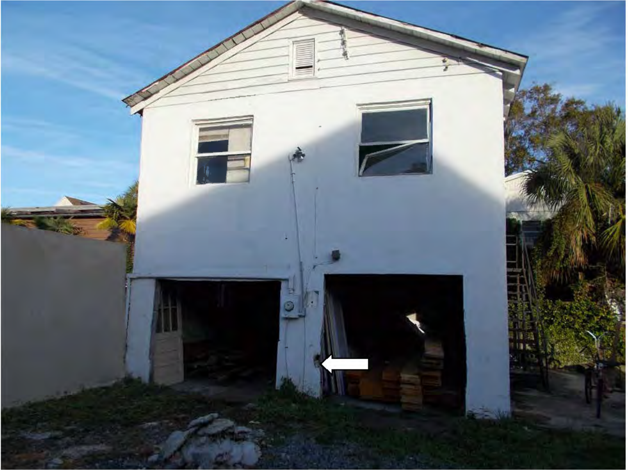
Figure 1: South Façade of the 66 Cannon Street ADU. Note the damage to the CMU at the opening
