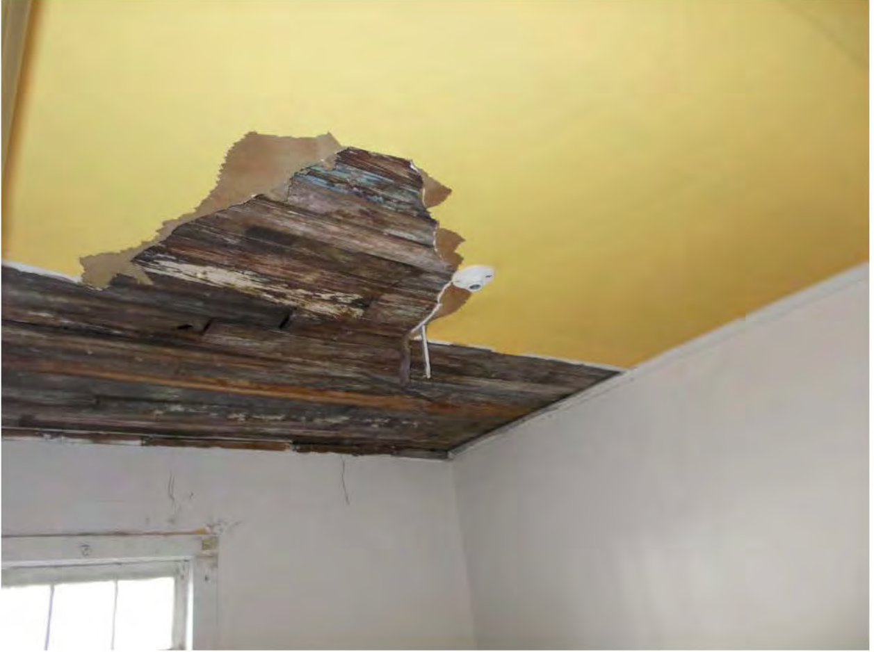
Figure 8: west side second floor ceiling water damage
