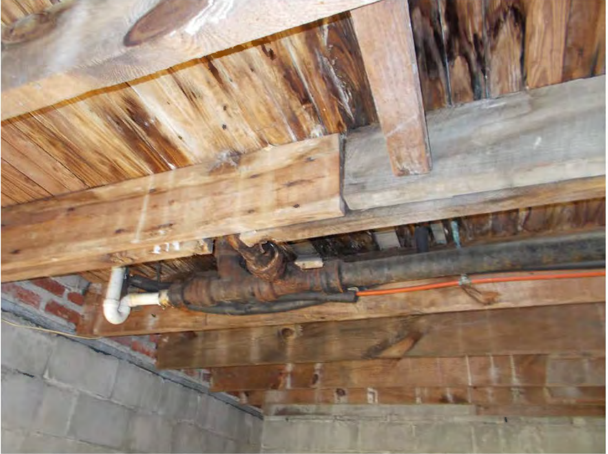
Figure 7: Second floor framing under the bathroom, showing deteriorated framing and inadequate framing supplementation.
