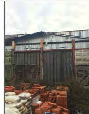
THE STRUCTURE OF GABLE ROOF AT THE INSIDE FACE OF THE EXISTING EAST ELEVATION
